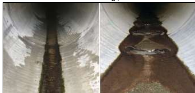
Flexi baffles in this culvert have created deeper, slower water flow to help fish pass through.
