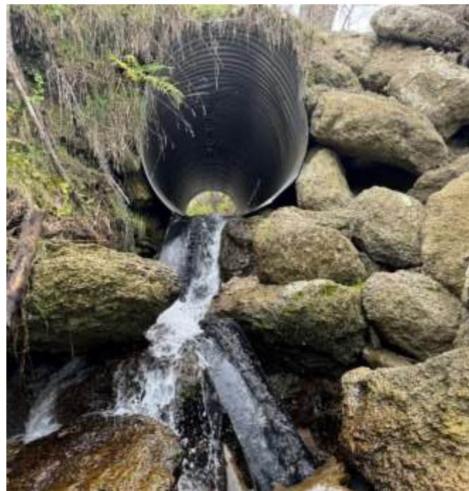
This Burden Road culvert was scoured out during cyclone Gabrielle. Some conveyor belt and mussel spat rope will help climbing species like eels and banded kokopu get up and into upstream habitat
